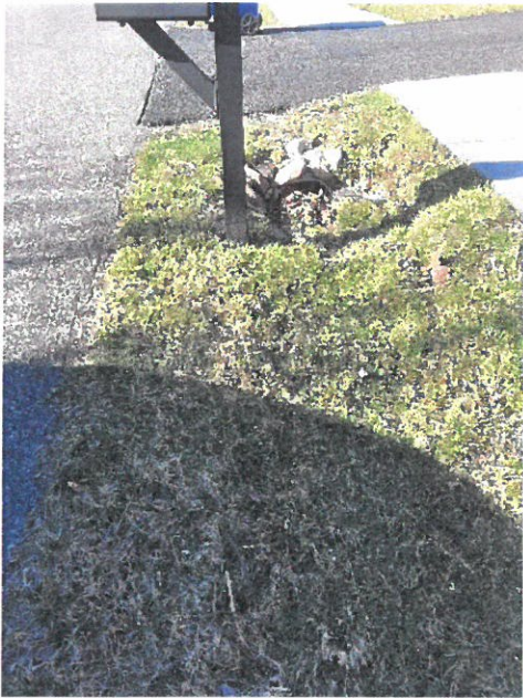
Clogged driveway outlet pipe – no ditch
