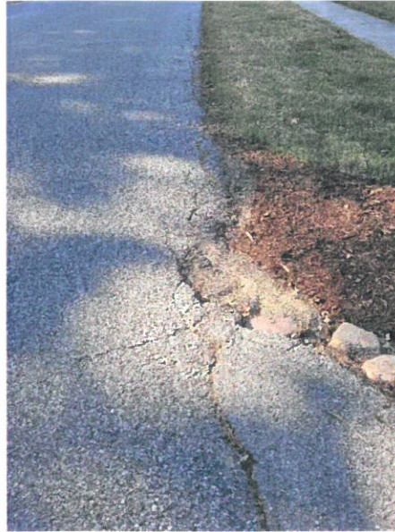
Stormwater damage along roadside
