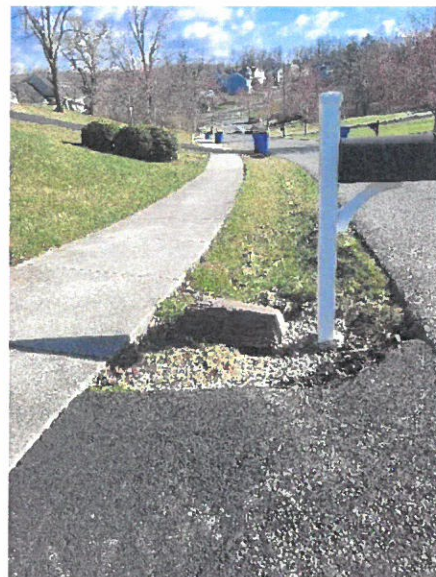
Driveway outlet crushed and buried
