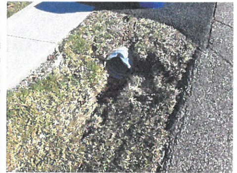
Driveway inlet culvert with road and sidewalk damage
