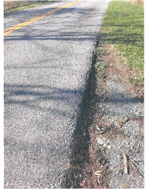
Erosion and damage along roadside
