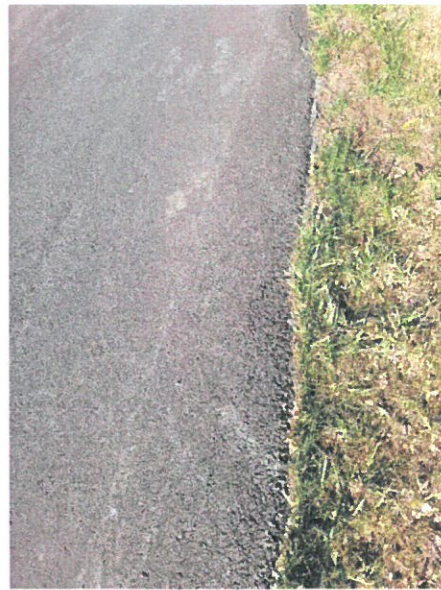
Edge cracking on brand new road surface installed fall 2022
