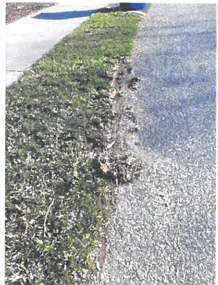
Damage to median due to lack of curbing
