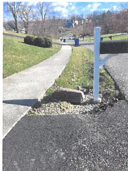
Driveway outlet crushed and buried
