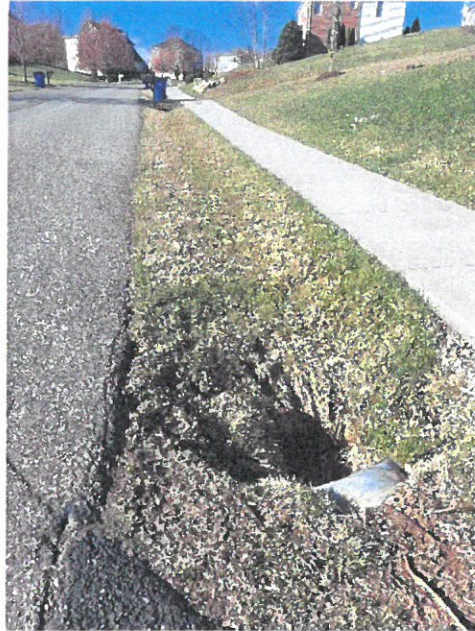
Driveway inlet culvert – Ditch filled in
