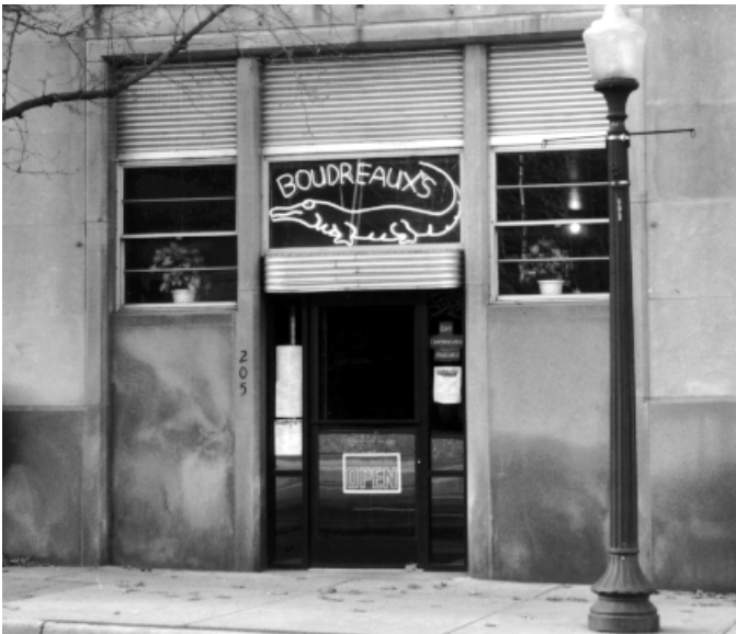
An example of innovative use of prefabricated material -- corrugated metal. These original metal infill panels are consistent in scale and quality with downtown commercial buildings
