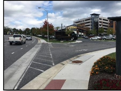
Faded, non-compliant pavement markings
