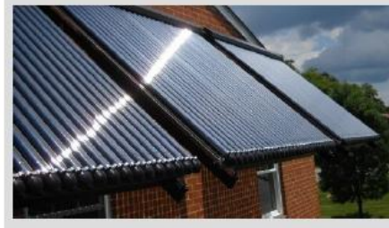
Above: The Solar Hot Water System installed by Dave Roper at his apartment building on Broce Drive. A wealth of other details on Dave's Solar Water Heating array (and pretty much any other energy topic) can be found at his blog: http://www.roperld.com/science/SolarHotWaterApartmentHouse.htm
